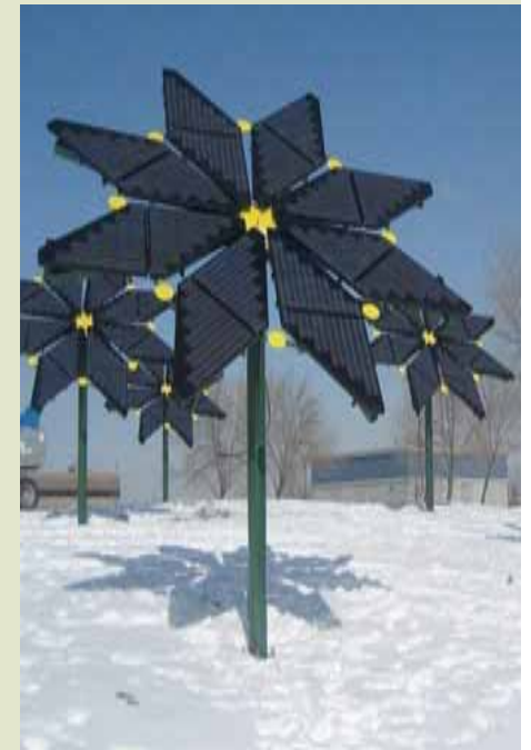
Solar Flair, installed by Lake Michigan Wind and Sun
